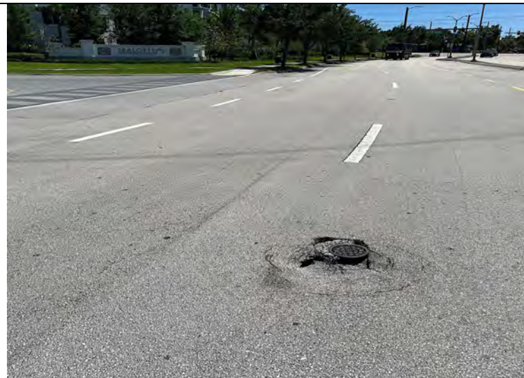
Photo 30: Asphalt around Valve Box needs Repair RCBN
