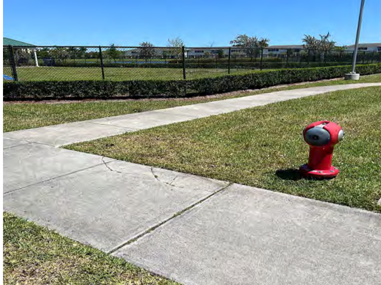
Photo 13: Broken sidewalk SW corner of south dog park on RCBN
