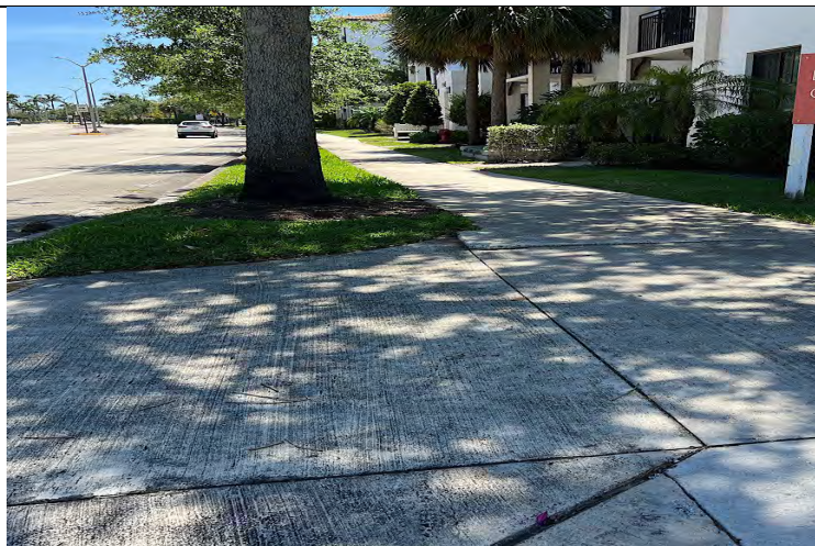
Photo 21: Trip Hazard in Sidewalk RCBS
