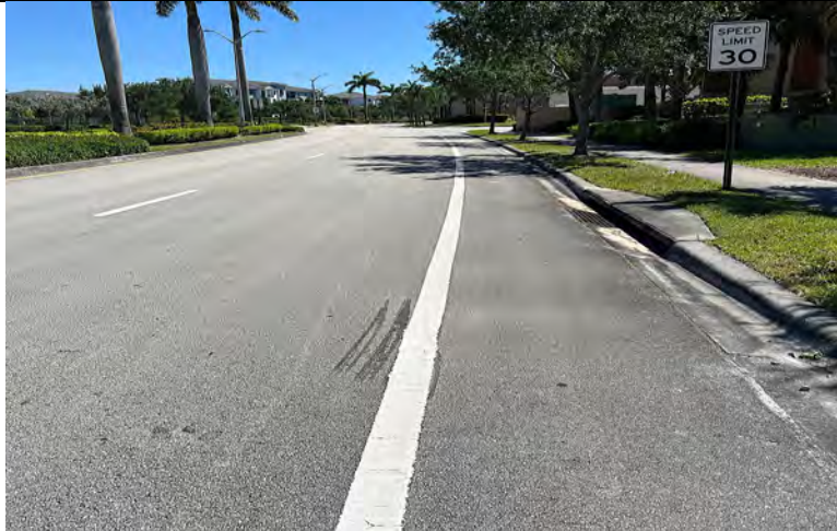
Photo 22: Gouges in Pavement RCBS
