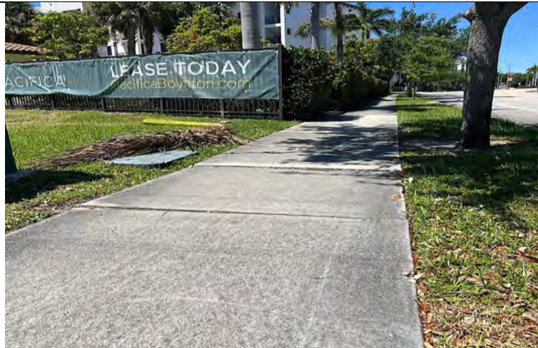
Photo 20: Trip Hazard in Sidewalk RCBS
