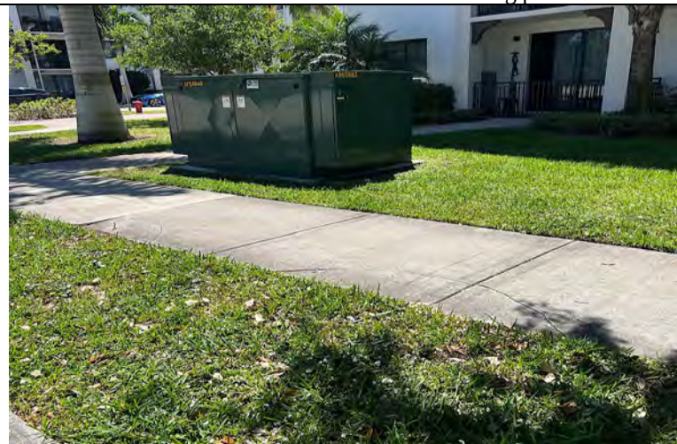
Photo 15: Broken sidewalk north of Audace Avenue on RCBS
