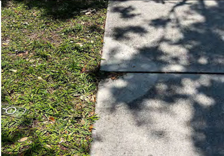
Photo 17: Chipped areas of sidewalk on RCBN
