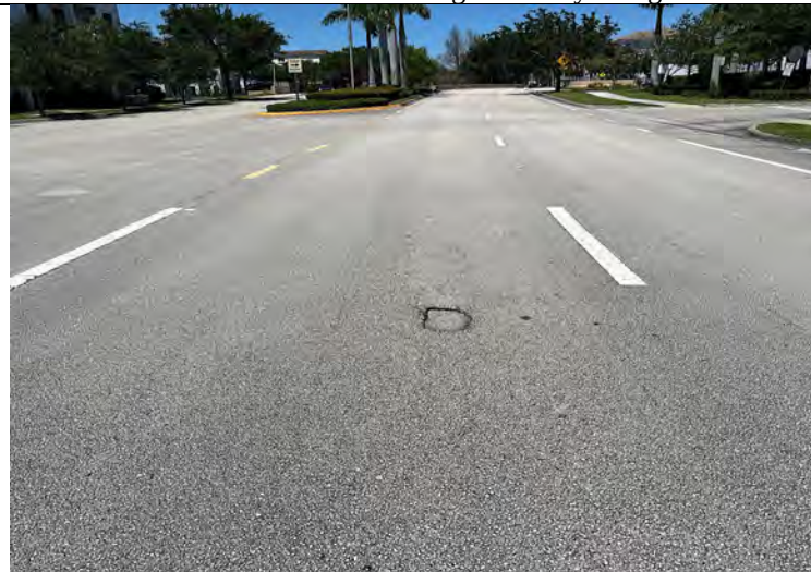
Photo 32: Pothole forming RCBN by Bridge
