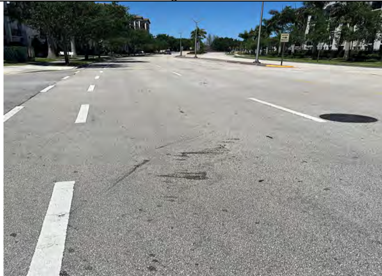
Photo 23: Gouges in Pavement RCBS
