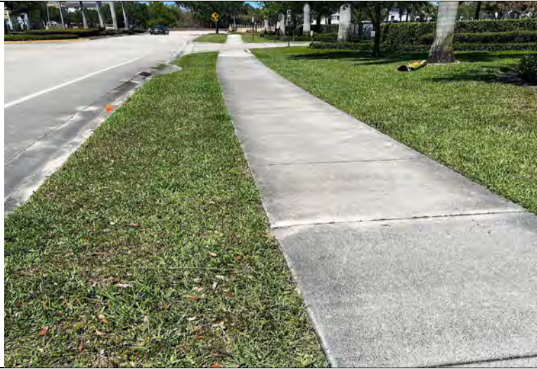
Photo 19: Chipped Sidewalk-Trip Hazard RCBN
