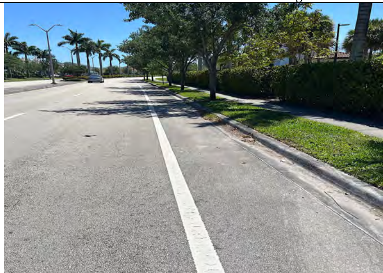
Photo 27: Dirt in Gutter RCBS South of Audace Ave
