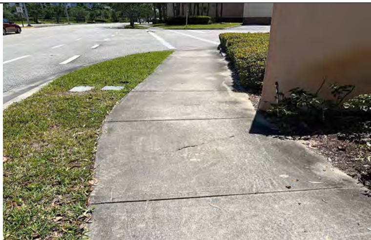
Photo 12: Broken sidewalk behind Michaels on RCBS
