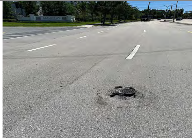
Photo 30: Asphalt around Valve Box needs Repair RCBN
