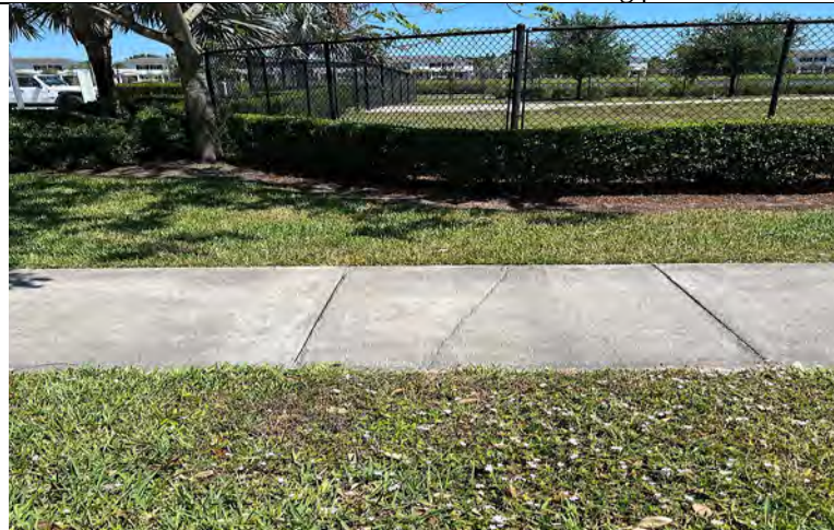
Photo 14: Broken sidewalk NW corner of south dog park on RCBN
