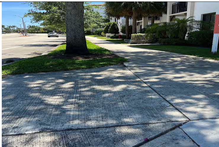
Photo 21: Trip Hazard in Sidewalk RCBS
