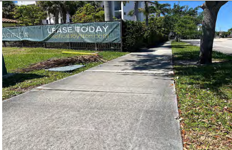
Photo 20: Trip Hazard in Sidewalk RCBS
