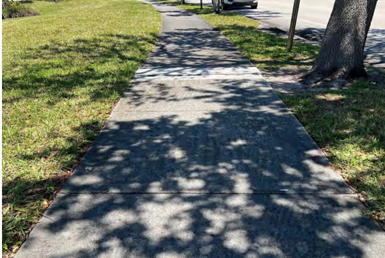
Photo 16: Trip hazard in sidewalk on RCBS
