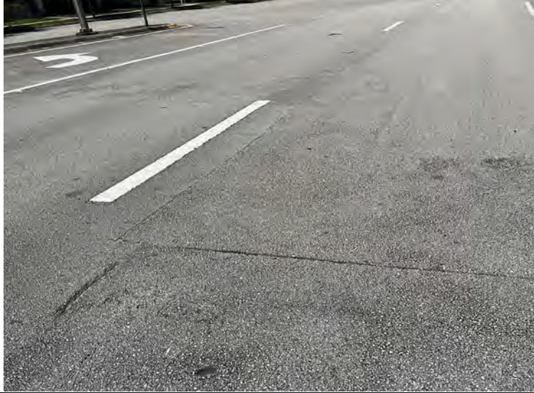
Photo 31: Pothole forming RCBN by Bridge
