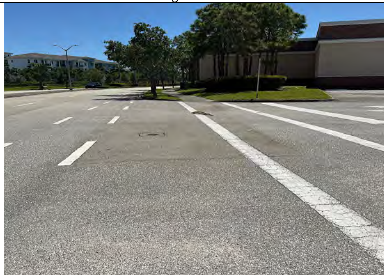
Photo 24: Ponding in Asphalt by Target Entrance
