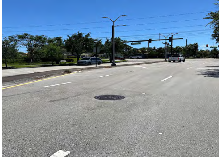
Photo 25: Dirt in Gutter RCBS by Old Boynton Road
