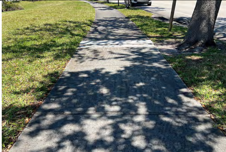
Photo 16: Trip hazard in sidewalk on RCBS
