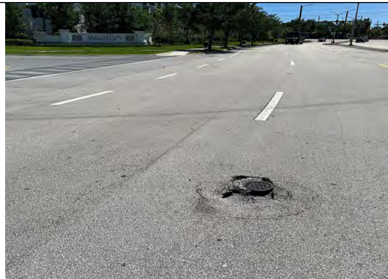
Photo 30: Asphalt around Valve Box needs Repair RCBN
