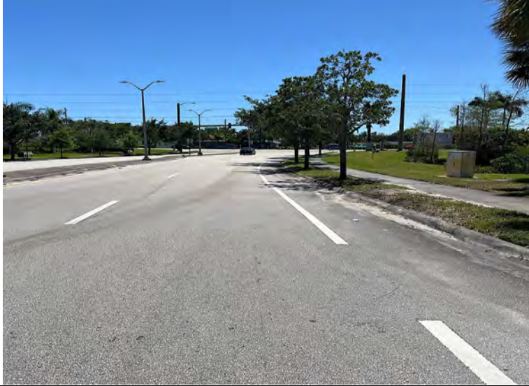
Photo 28: dirt in Gutter RCBS west side by Old Boynton Rd
