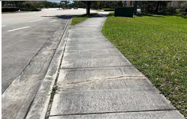
Photo 11: Broken sidewalk in bus dropoff area on RCBS.
