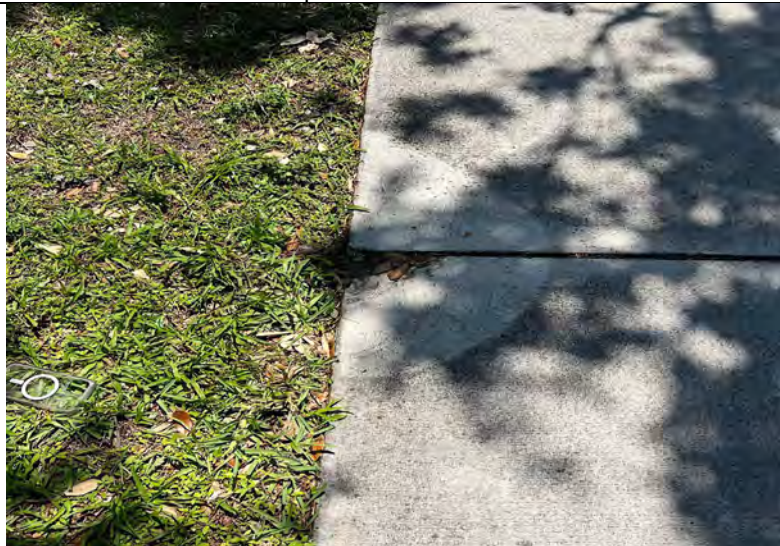
Photo 17: Chipped areas of sidewalk on RCBN
