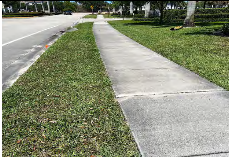
Photo 19: Chipped Sidewalk-Trip Hazard RCBN
