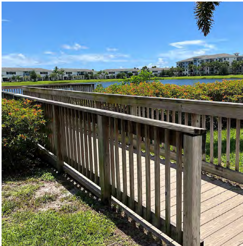
Photo 46: Observation Deck top rail starting to warp
