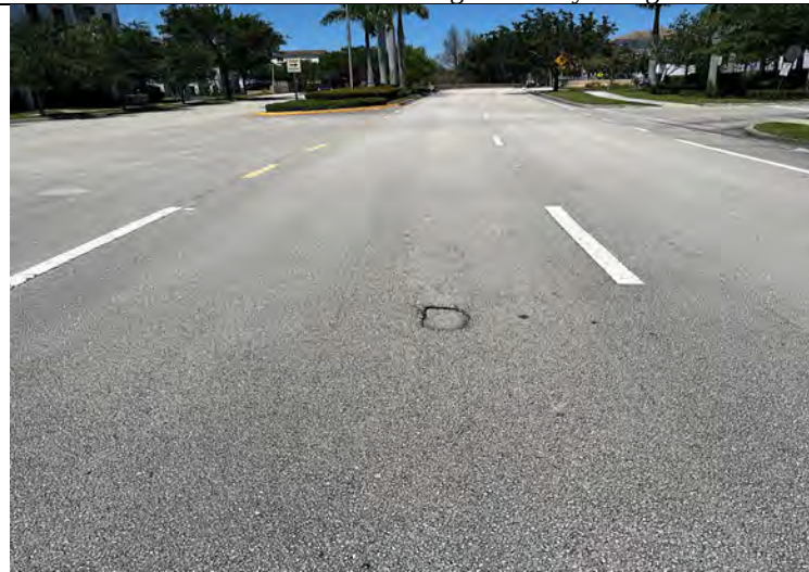
Photo 32: Pothole forming RCBN by Bridge
