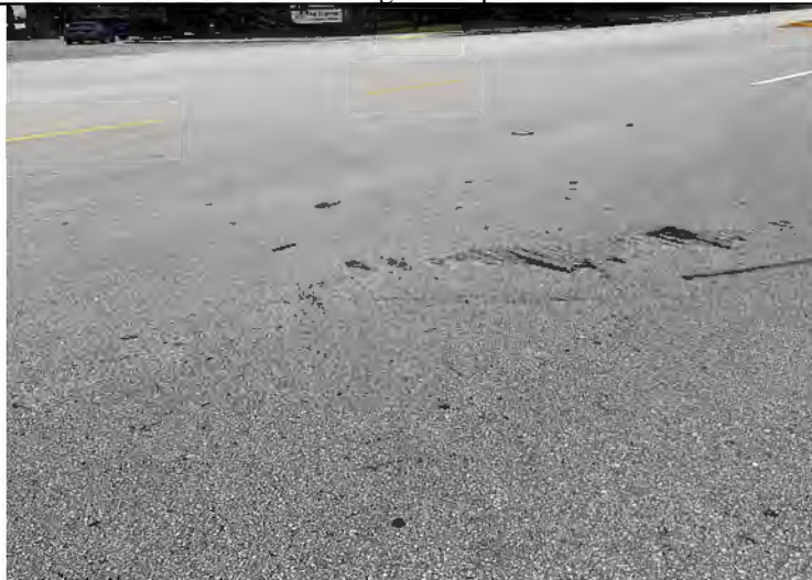
Photo 29: Gouges in road RCBS
