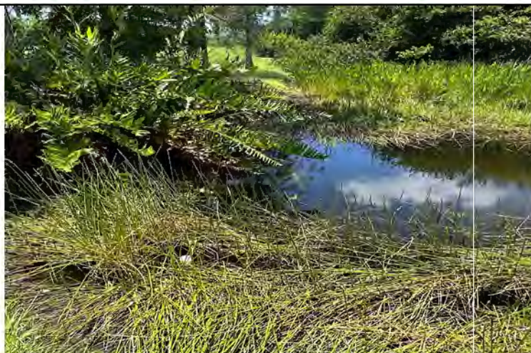
Photo 6: Steep Slope sign missing-outfall needs excavation
