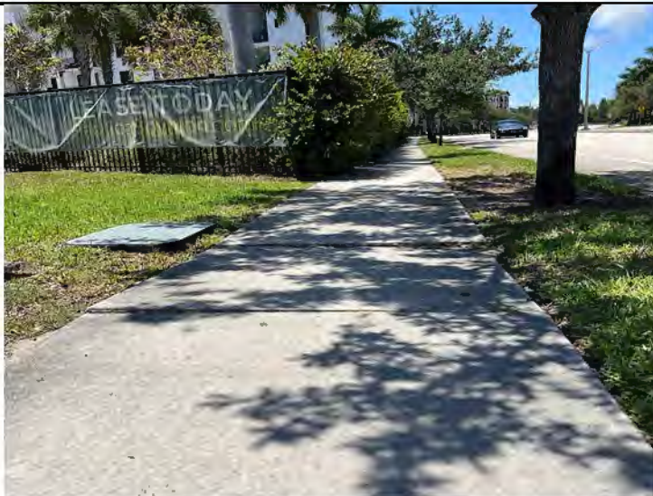
Photo 24: Trip hazard in walk-bushes blocking walk south of Audace Ave RCBS
