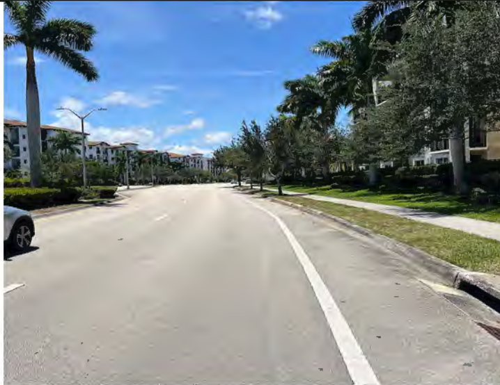
Photo 34: RCBN-dirt in gutter south of The District
