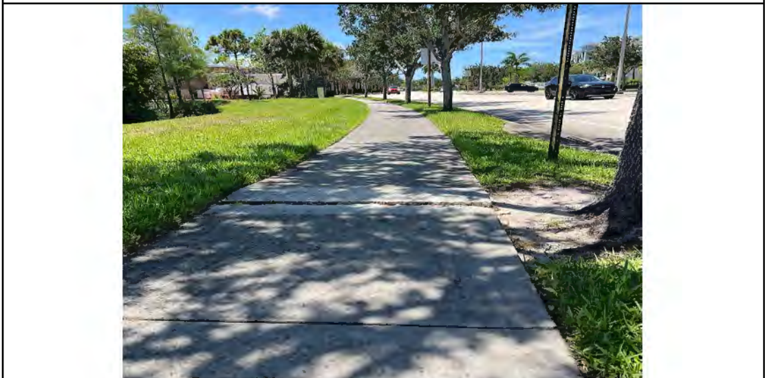
Photo 27: Trip hazard in walk-several areas RCBS
