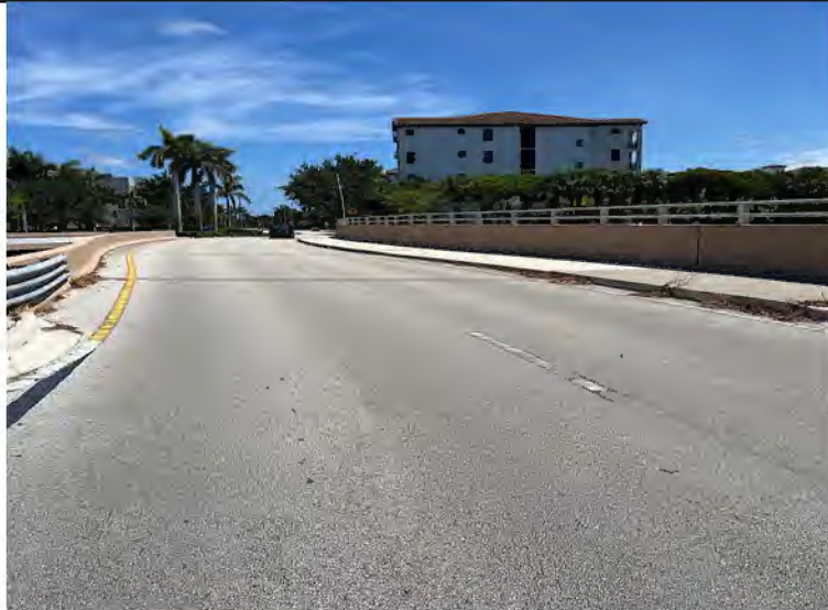
Photo 40-RCBS-dirt and weeds on bridge
