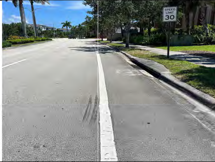
Photo 28: Gouges in asphalt RCBS
