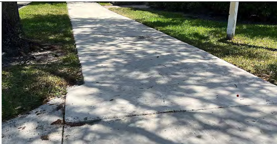
Photo 21: Trip Hazard-broken Walk south of bridge RCBS
