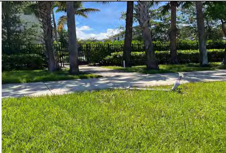
Photo 43: Greenway-broken bollard light SE side
