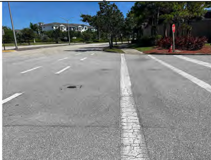
Photo 30: Ponding of water at Target entrance RCBS
