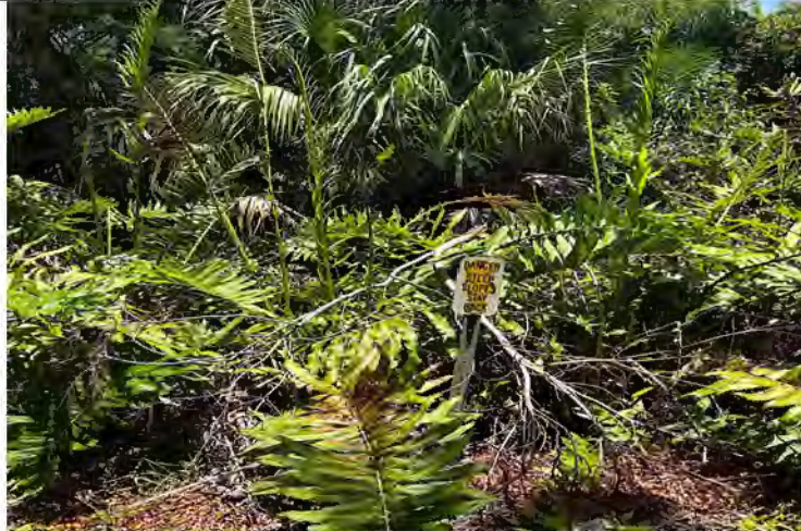
Photo 4: Steep bank-outfall pipe buried-needs excavation/extension.
