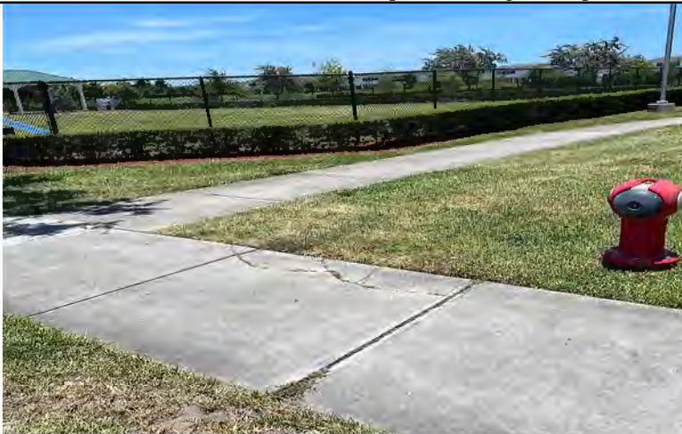
Photo 14: Broken sidewalk SW corner of south dog park on RCBN
