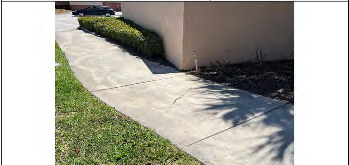
Photo 26: Broken walk behind Michaels RCBS
