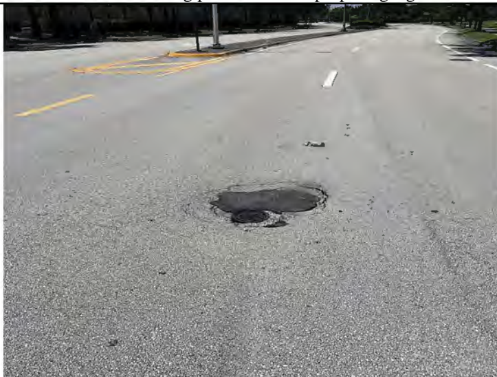
Photo 36: Asphalt repair needed by Sea Lofts on RCBN
