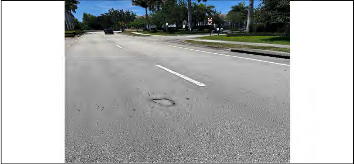
Photo 37: RCBN-pothole forming just south of bridge
