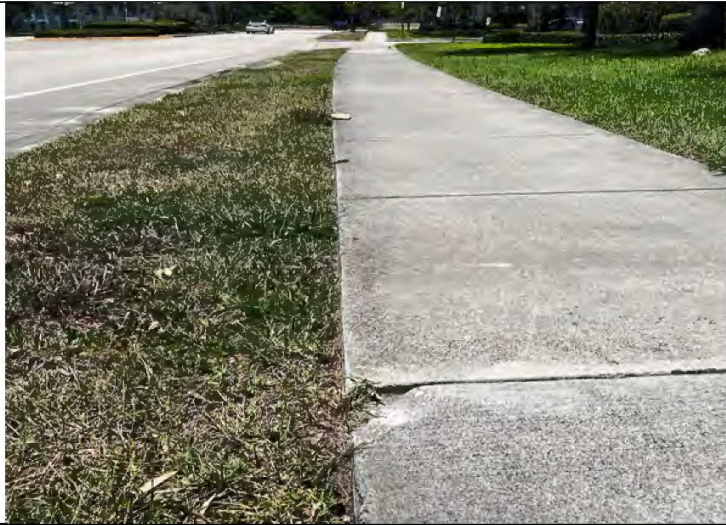
Photo 19: Chipped Sidewalk-Trip Hazard RCBN north of The District
