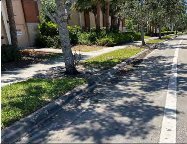
Photo 31: Dirt in gutter behind Michael RCBS
