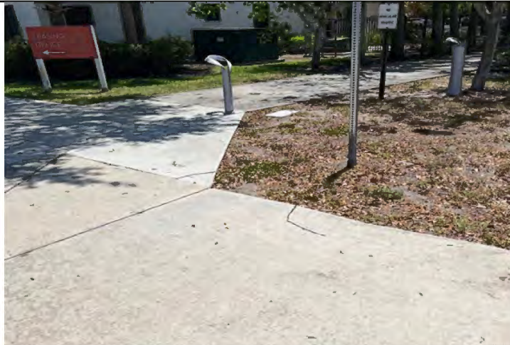
Photo 20: Broke Sidewalk-Trip Hazard south of bridge RCBS
