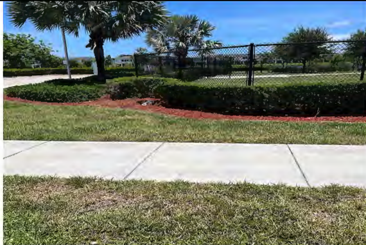
Photo 15: Broken sidewalk NW corner of south dog park on RCBN
