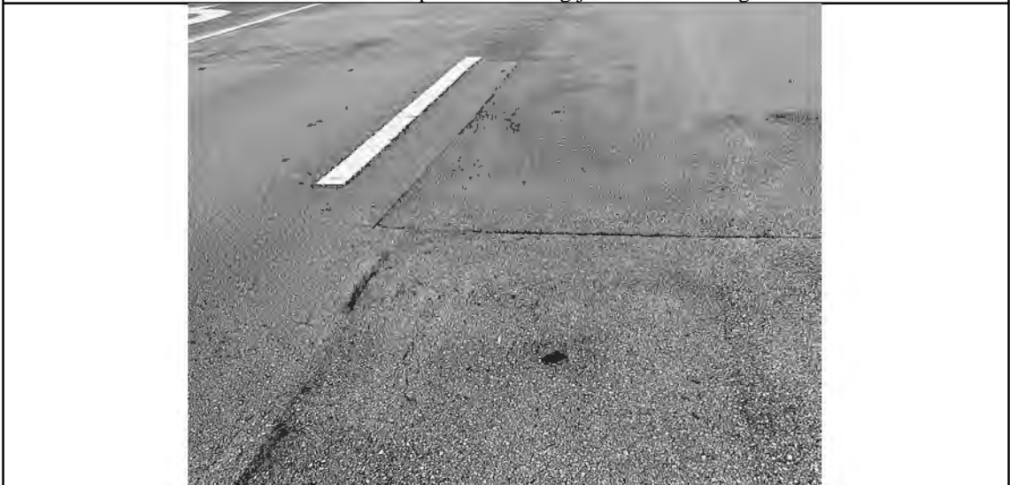
Photo 38: RCBS- small holes forming just south of bridge
