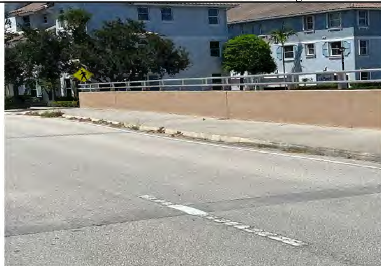
Photo 41-RCBN-dirt and weeds on bridge
