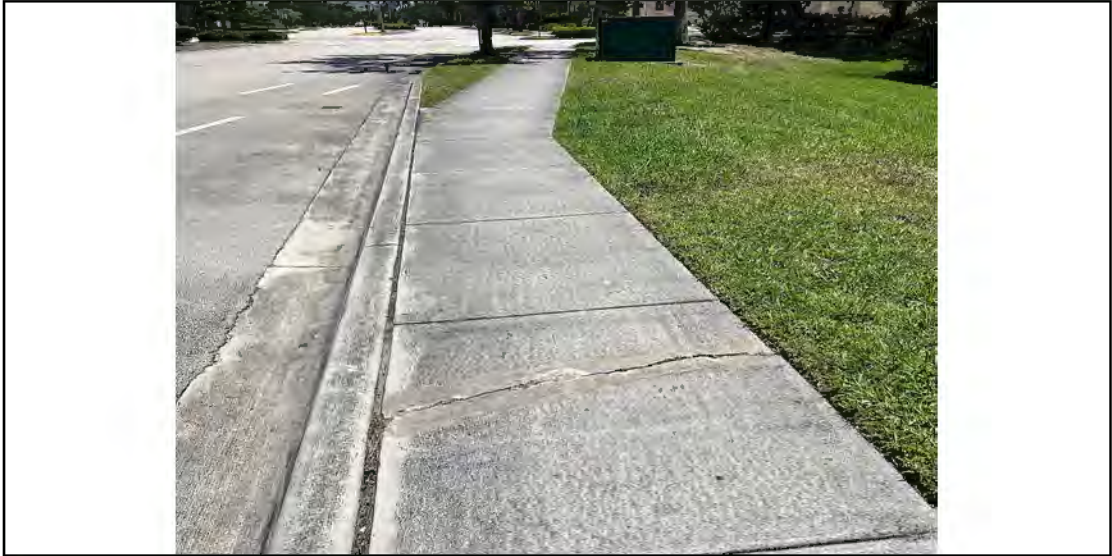
Photo 25: Broke walk in bus drop-off RCBS
