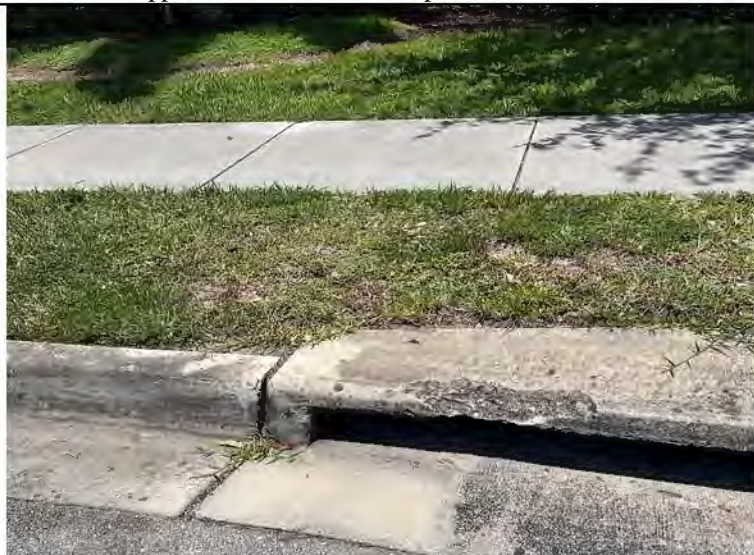
Photo 18: Chipped inlet top should be patched on RCBN.
