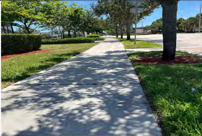
Photo 16: Trip hazard in sidewalk south of north dog park on RCBN
