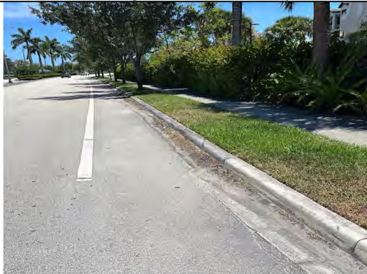
Photo 33: Dirt in gutter RCBS south of Audace Ave
