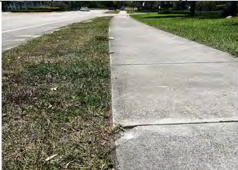
Photo 17: Chipped areas of sidewalk-trip hazard on RCBN north of dog parks
