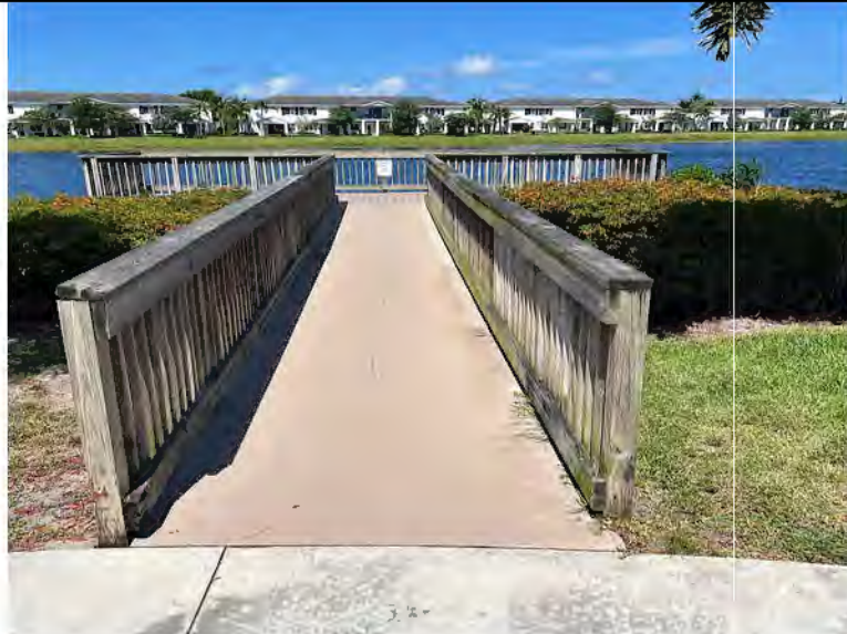
Photo 13: Observation deck top rail starting to warp
